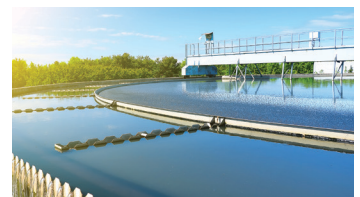
Water and Wastewater Systems
